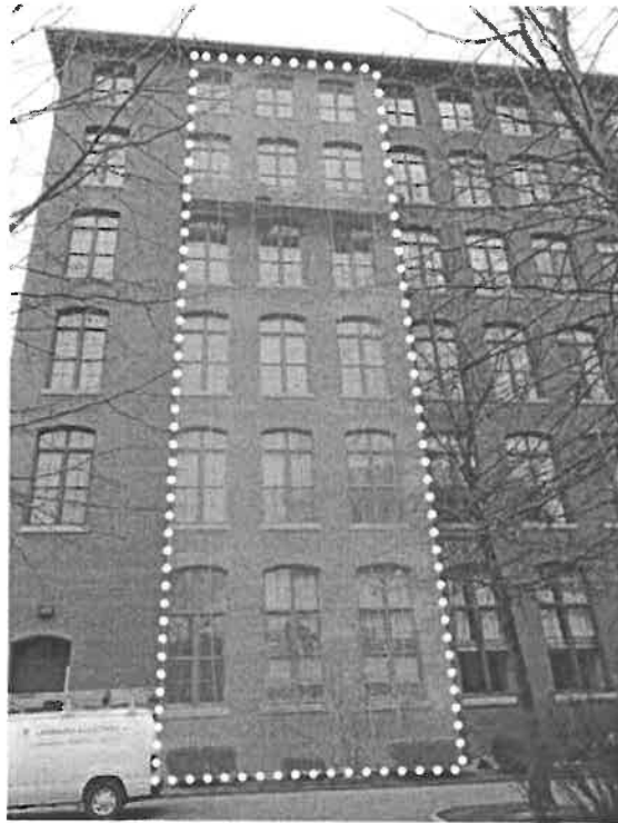
Photograph 1 – The masonry in the 1 st staging drop is located within the dotted rectangle.
