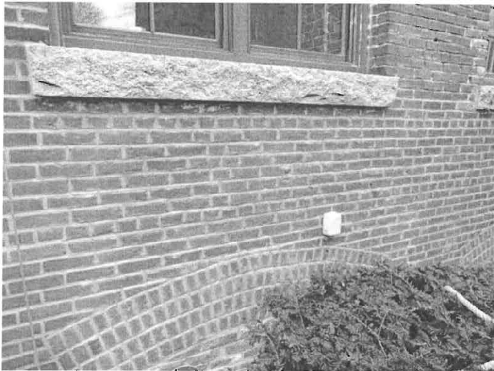
Photograph 2 – Newly pointed mortar joints at the base of the 1 st staging drop.
